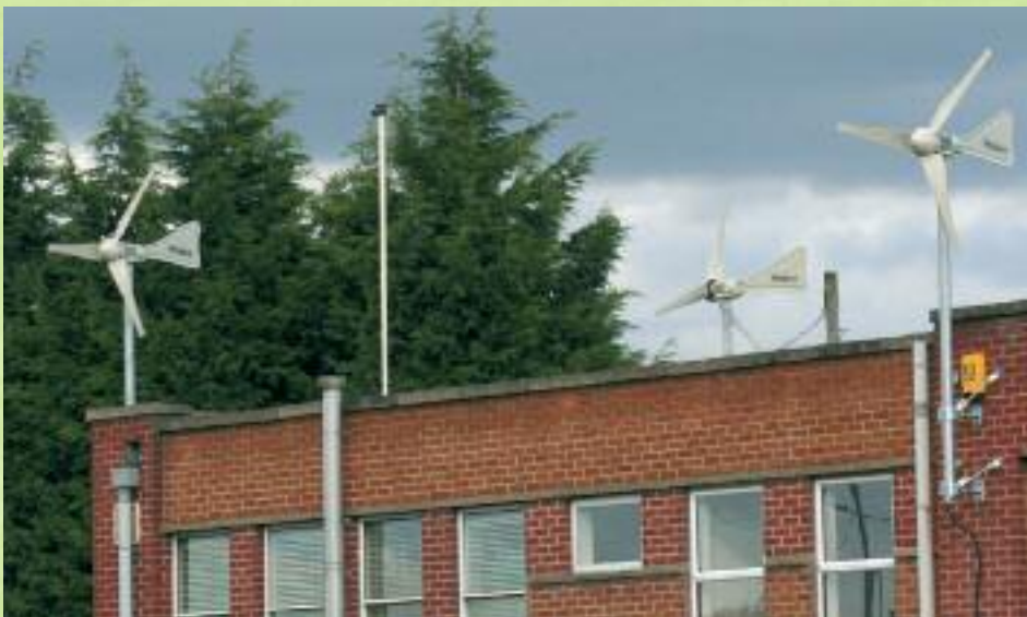
Three wind turbines on the roof of the Ecoskies training centre in Chesterfield.
